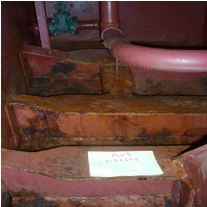
Figure 1 Corrosion Under Insulation (CUI): Corrosion under conventional lagging system on the USS Crommelin Photo Courtesy of US Navy
