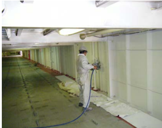
Figure 7 Commercial Application of TEMP-COAT 101 to stop condensation issues and associated mold growth aboard car carrier Asian Spirit. Photo Courtesy of Nissan Fleet Operations
