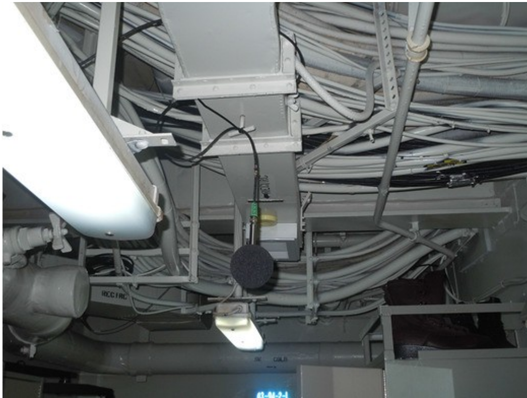
Figure 5. Microphone installation in stateroom
