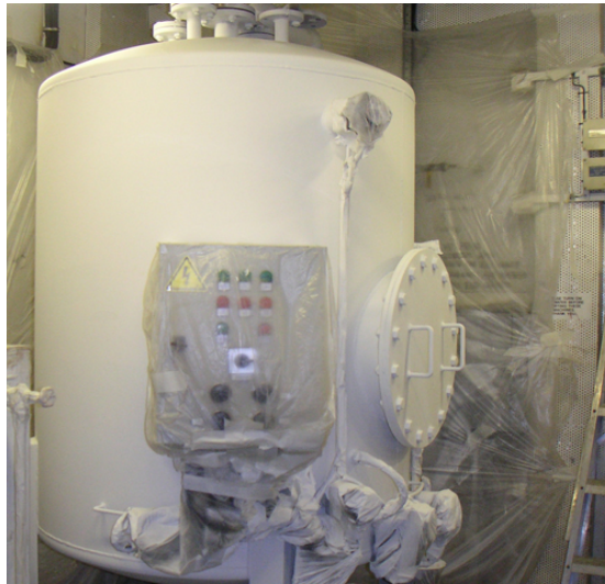
Figure 5 Application of TEMP-COAT 101 Insulation Coating on hot oil tank for personnel protection and energy savings aboard the RFA Fort George Photo Courtesy of British Navy
