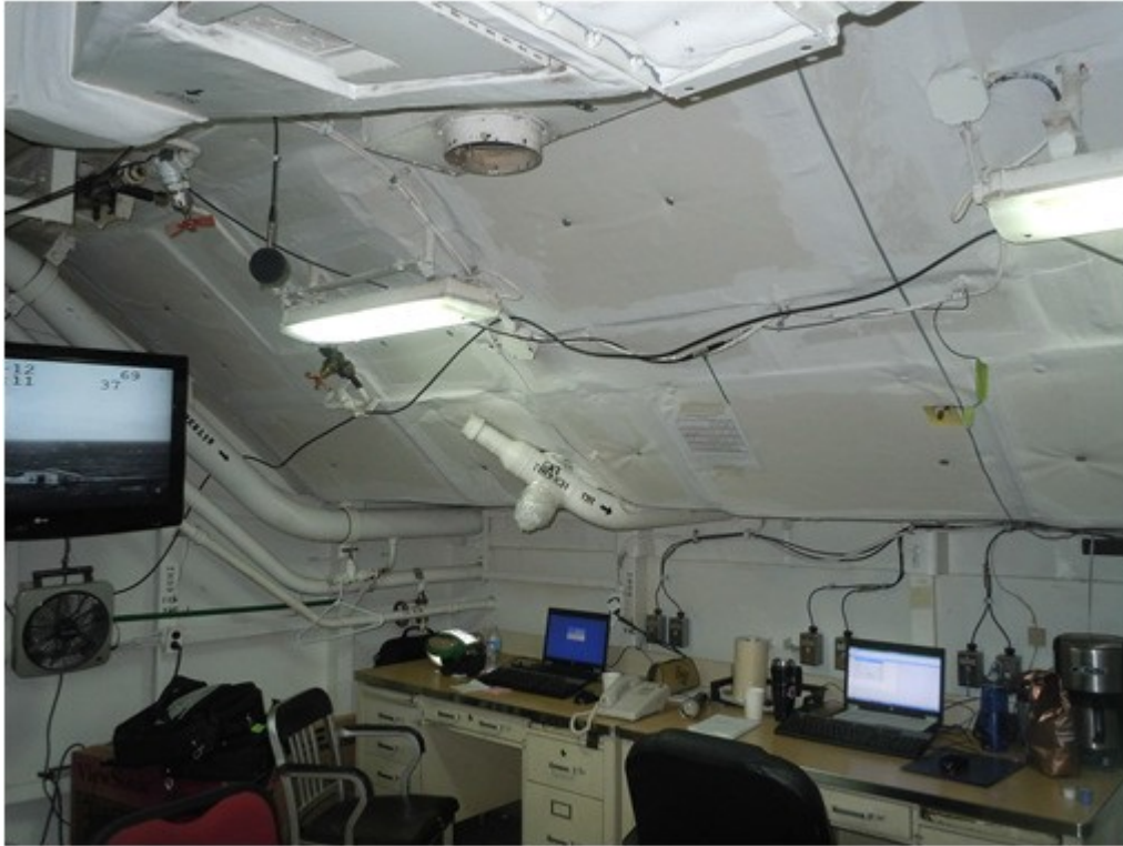
Figure 10. Microphone and accelerometer installation in maintenance office
