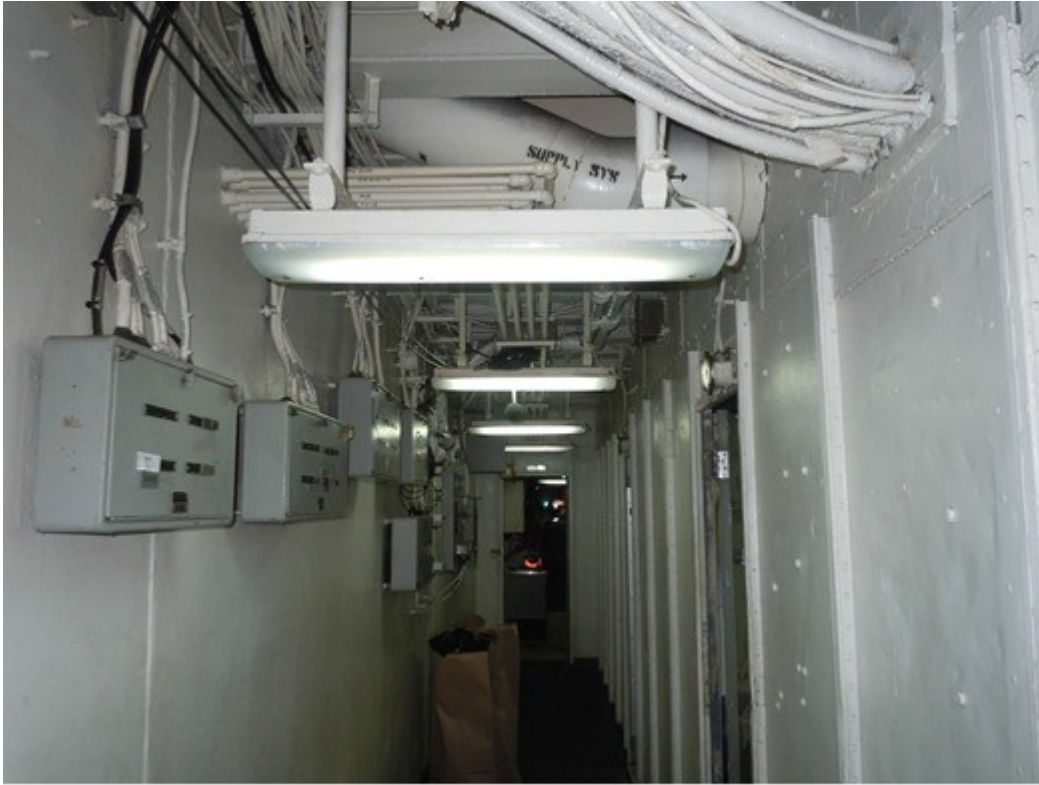
Figure 4. Microphone installation in passageway
